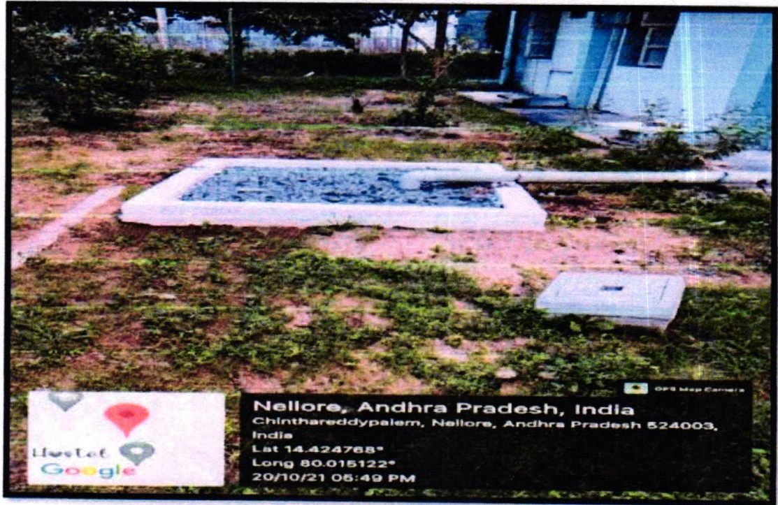
Fig.1: Rain Water Harvesting (RWH) system implemented in the College
